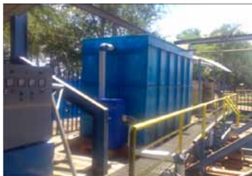
Gambar 2. Pilot plant biofiltrasi di Intake Taman Kota
