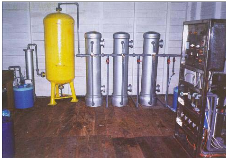
Gambar 6. Peralatan Unit RO, Filter dan Reaktor Tank
