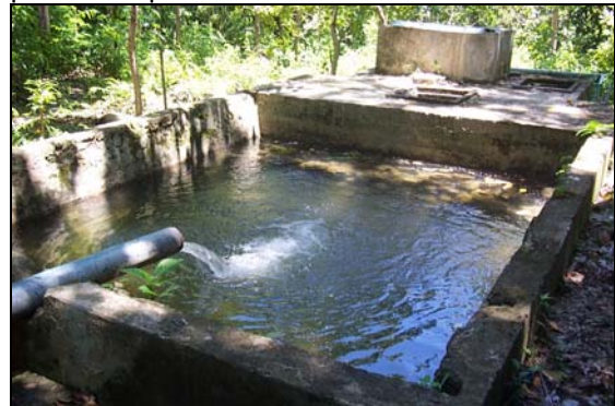
Gambar 4. Bak Saringan Pasir Lambat Somba Eksisting
